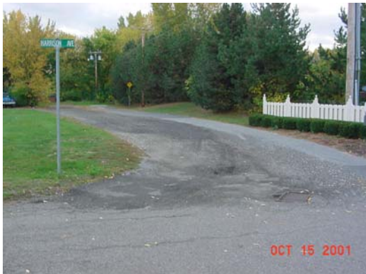
Figure 1: It is difficult to tell where path begins and driveway ends. Further delineate this difference to improve safety.
