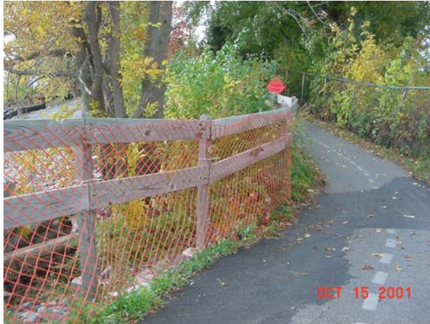
Figure 6: Poor visibility north of Barge Canal Bridge
