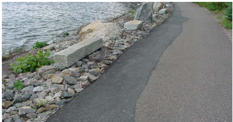
Figure 7: Erosion at riprap wall
