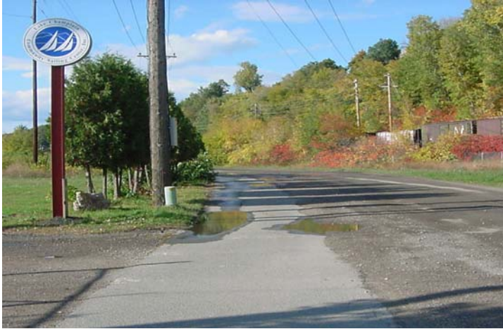
Figure 8: Path intersects with Sailing Center Drive - Ponding Evident
