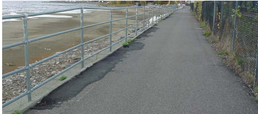
Figure 5: Path erosion near Barge Canal Beach
